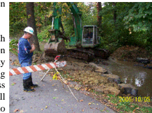
Workers begin installing the Rock "vaness" along the Tuscarora Creek at War Memorial Park in October.
